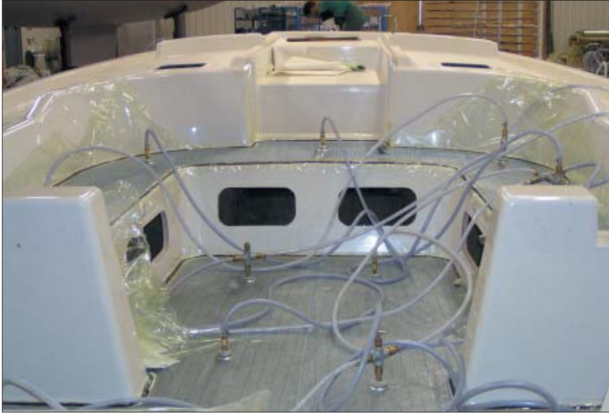
To avoid the use of fasteners and the inevitable problems with bungs and leaks, the teak decks on a Hanse 531 cockpit are vacuum-bagged in place.
